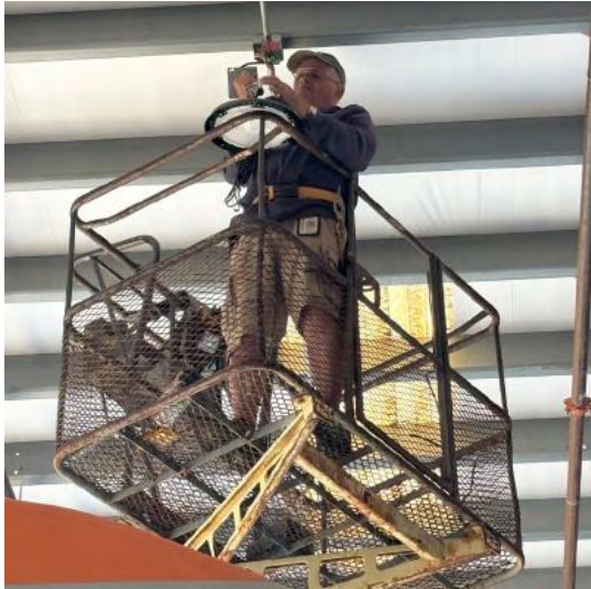
Roger Tonovitz replaces one of the metal halide hangar fixtures with an LED fixture.
