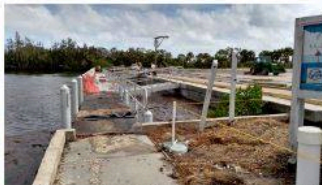
Bairs Cove boatramp being evaluated after Hurricane Irma Photo by MINWR Staff
