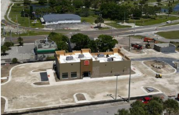
Site and building construction are nearing completion for a 3,117-square-foot drive-thru restaurant located along S. Washington Avenue near Garden Street.
