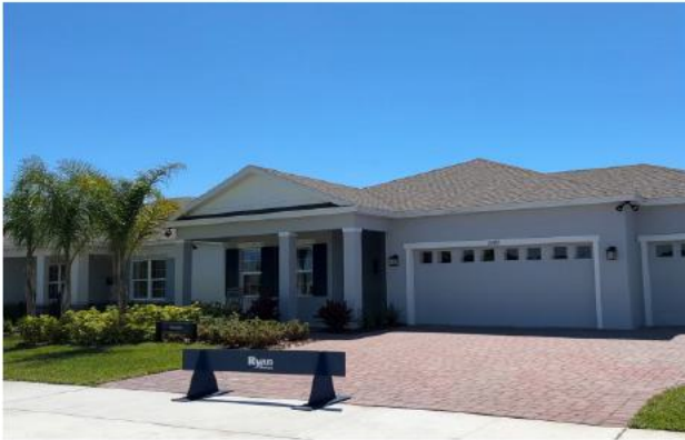
Site construction continues and houses are being built at a 143-unit single-family home subdivision located along Jay Jay Road.
