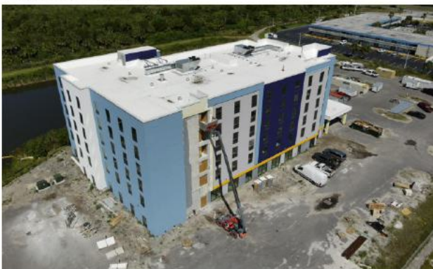
Site construction is nearly complete for a 68,992-square-foot, 122-room hotel located on South Helen Hauser Boulevard.
